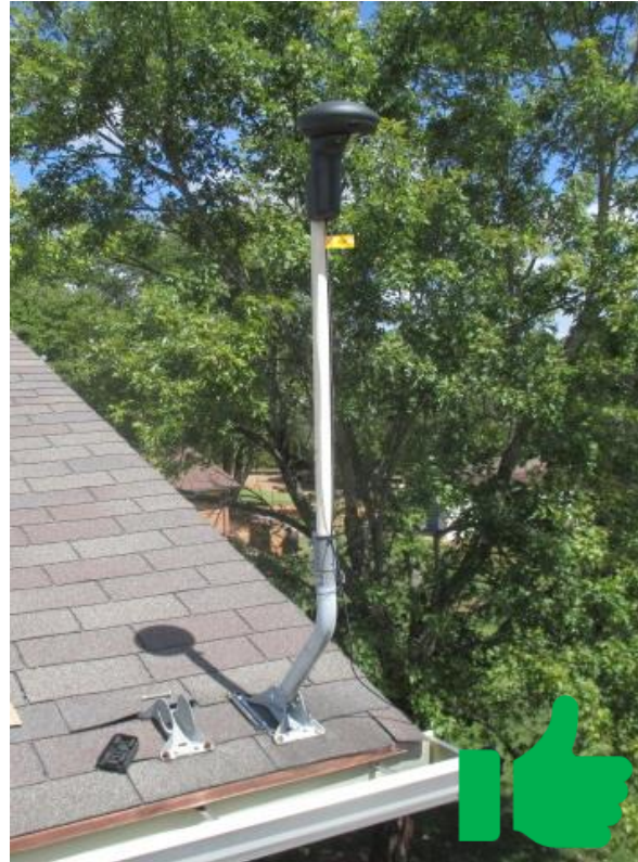
On roof utilizing existing Satellite TV mount. Raised to give plenty of clearance.
